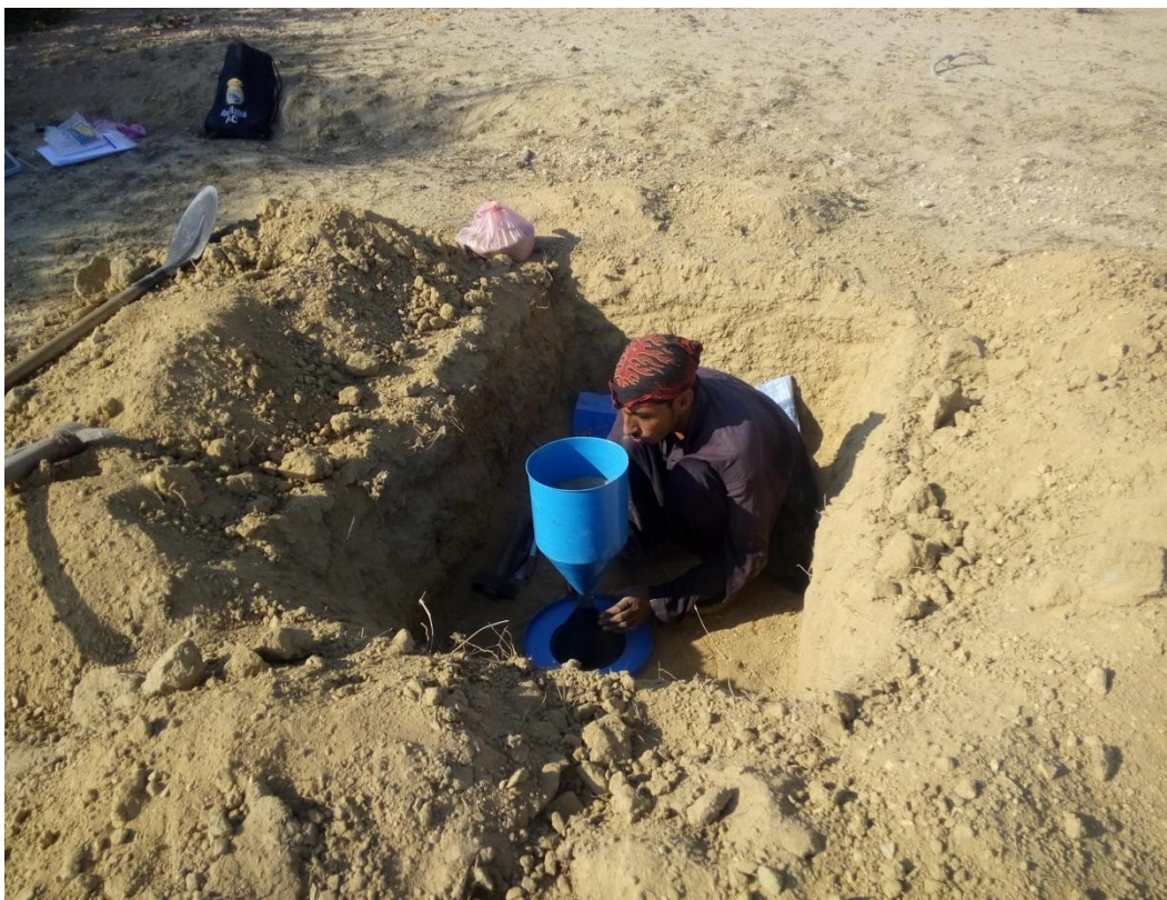
Performance of FDT at “Geotechnical Investigations for 50MW Tricom Wind Power Project, 347-Acres at Jhimpir, Sindh” Project
